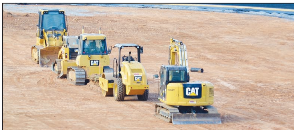
Heavy equipment operating last week on what used to be the Towns County football field, soon to be replaced with state-of-the-art artificial turf. Photo by Chad Stack
